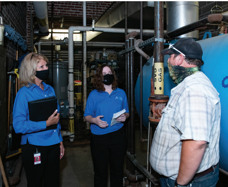
Steam trap replacements and boiler optimization were the keys to savings success for Donovan Junior/Senior High School.
