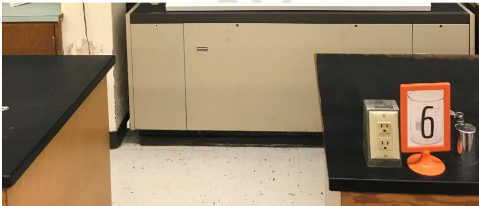
Figure 8: Classroom 205, Unit Ventilator had a Previously Undiscovered Air Leak between Left-hand Side of Cabinet Assembly and Structural Column
