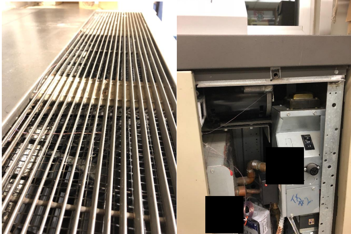
Figure 12: Classroom 203, Air Supply Thermocouple as Installed Prior to Baseline Period
