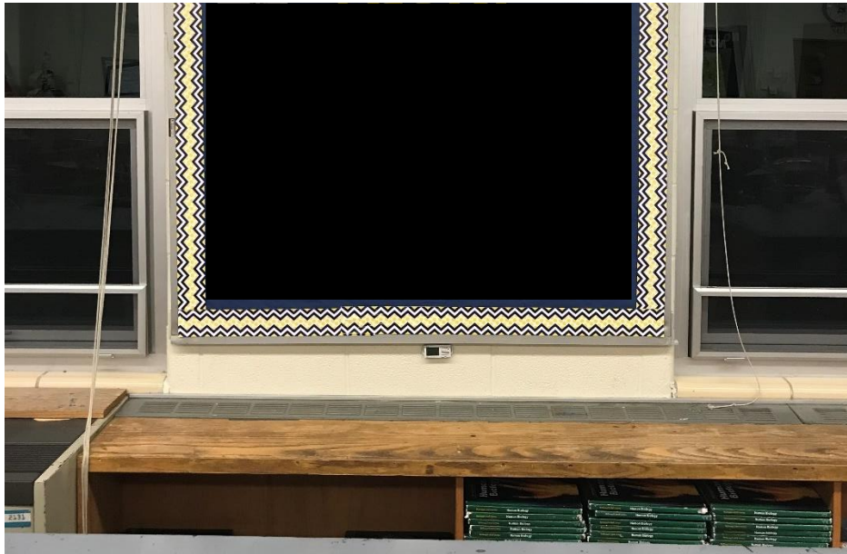
Figure 7: Classroom 137, Hidden Uncontrolled Radiator behind Bookshelf
