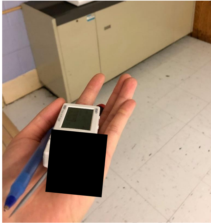
Figure 11: Classroom 147, South Unit Ventilator with a Maintenance Ticket for Grinding Fan Motors/Potential Motor Failure
