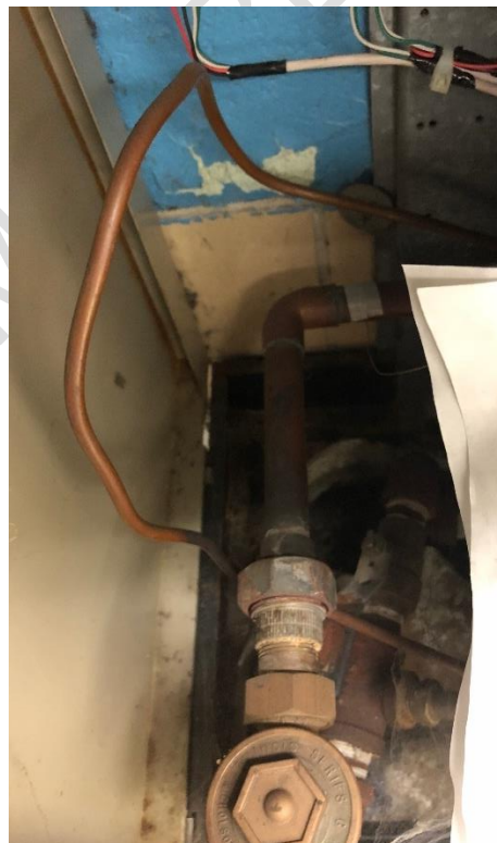
Figure 10: Classroom 147, Steam Leak Maintenance Ticket within North Unit Ventilator
