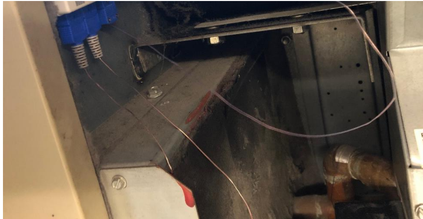
Figure 14: Classroom 203, Visible Break in Thermocouple Line below the Unit Ventilator Cabinet Entry-Point
