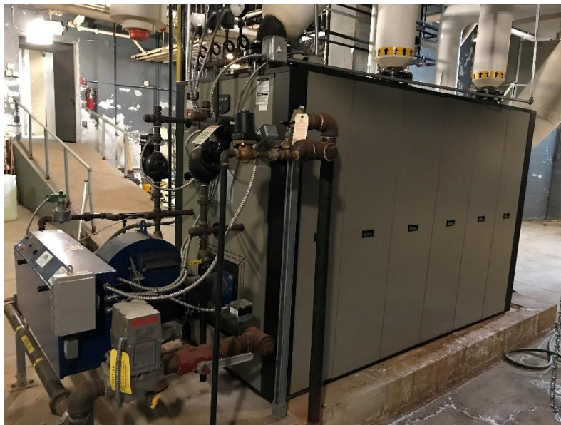
Figure 1 Steam Boiler serving the hydronic heating radiators
