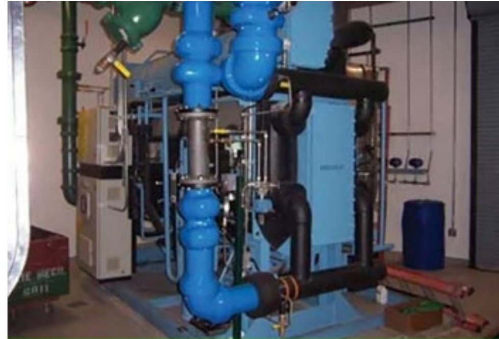
A 300-ton absorption chiller located at a data and research center at Syracuse University, New York. The chiller uses exhaust from twelve 65-kW microturbines and can cool water to 45°F. Photo courtesy of New York-New Jersey Onsite Energy Technical Assistance Partnership (TAP).
